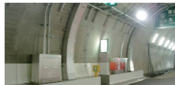
Fire extinguishing system for a tunnel on the Shinjuku Route of the Shuto Expressway where our stainless steel is used
